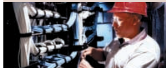
An Avnet Enterprise Solutions project engineer upgrades a customer's network infrastructure.
